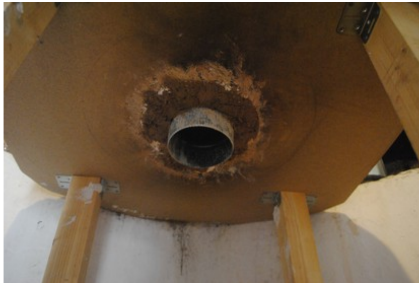
Figure 8. 15cm diameter pipe and 20cm long connecting the stove with the oven. Gaps sealed with mud with some plaster.
